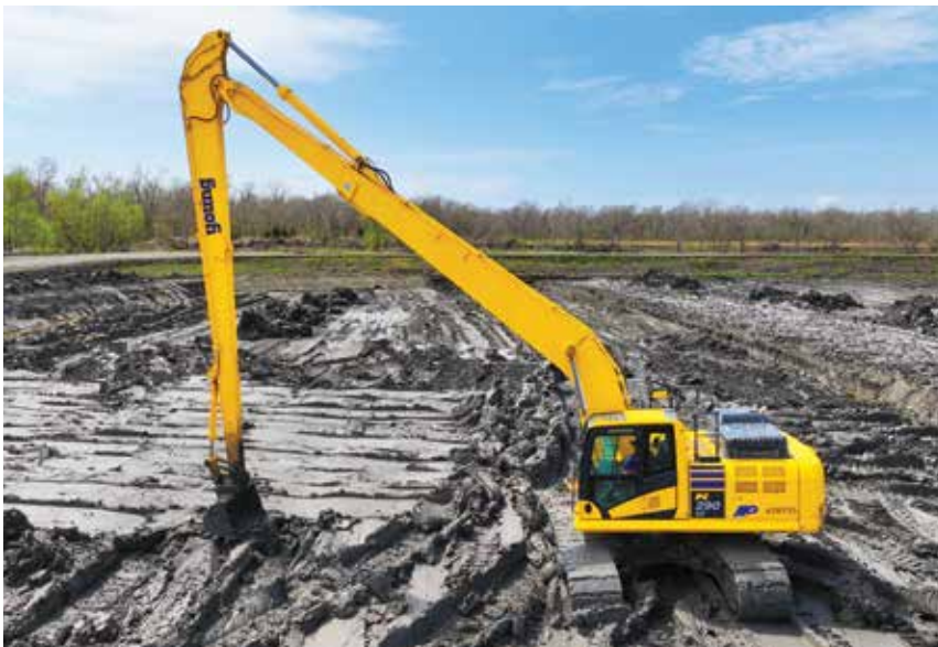
An operator digs material with a Komatsu PC290LC-11 long-reach excavator at Lirette Dirt Service's Chauvin, La., pit.
