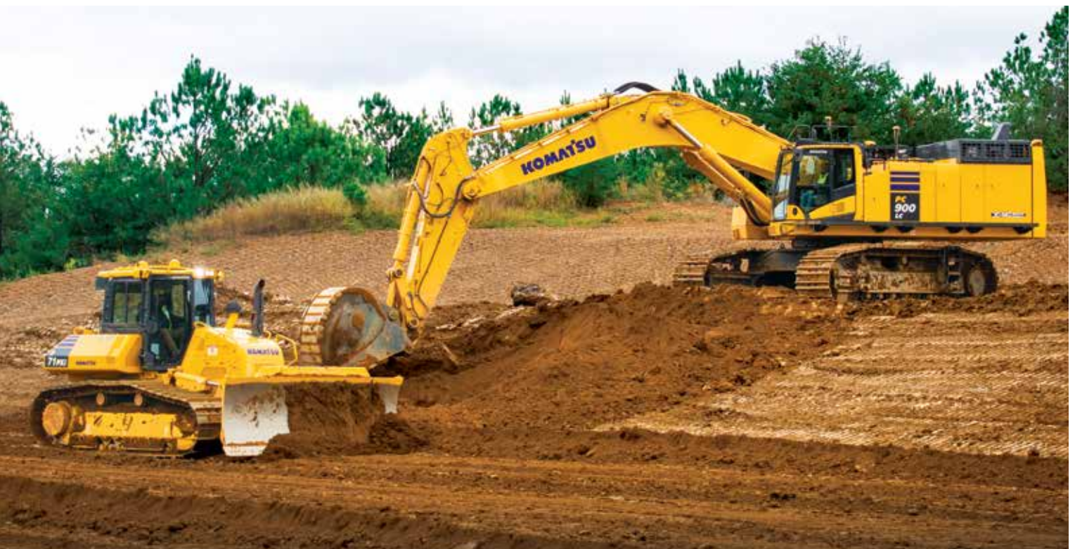
(L-R) WPI's Mark Bewley meets with Liles Crushed Concrete's Robin Liles and Dillon Liles at Demo Days.
