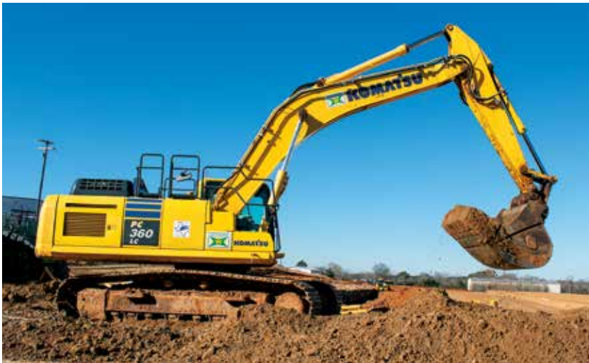
A W.R. Welborn & Son operator picks up material with a Komatsu PC360LC-11 excavator.
