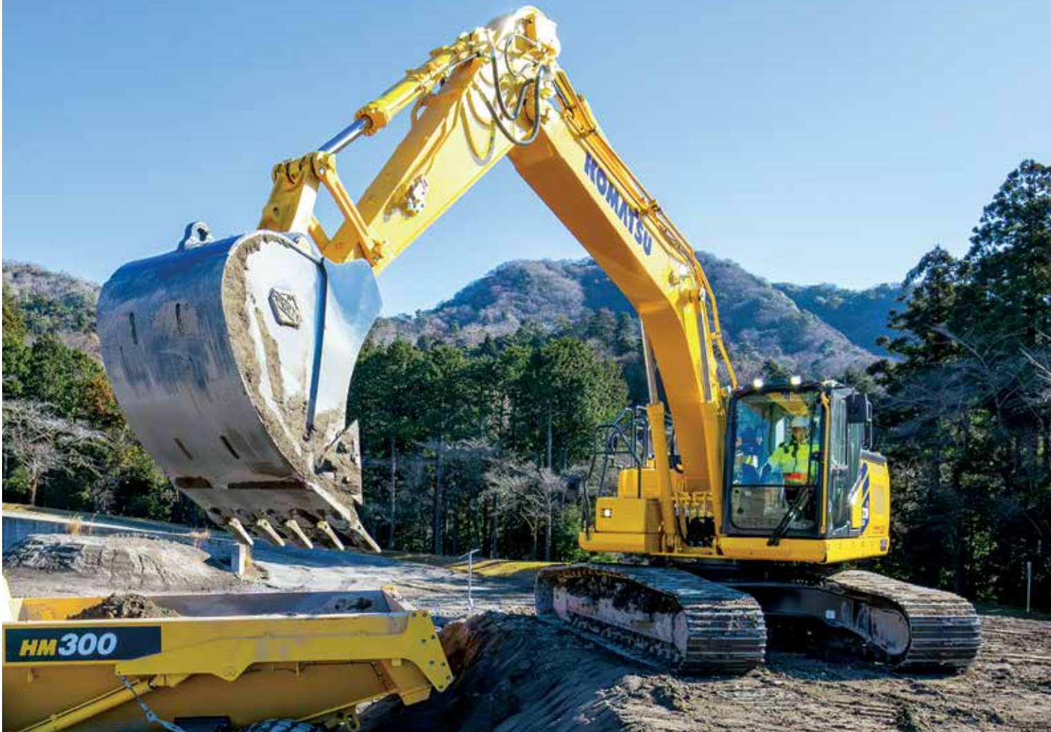
WPI's Smart Construction Services team helps customers use the latest technology such as Komatsu intelligent machine control (IMC) excavators.
