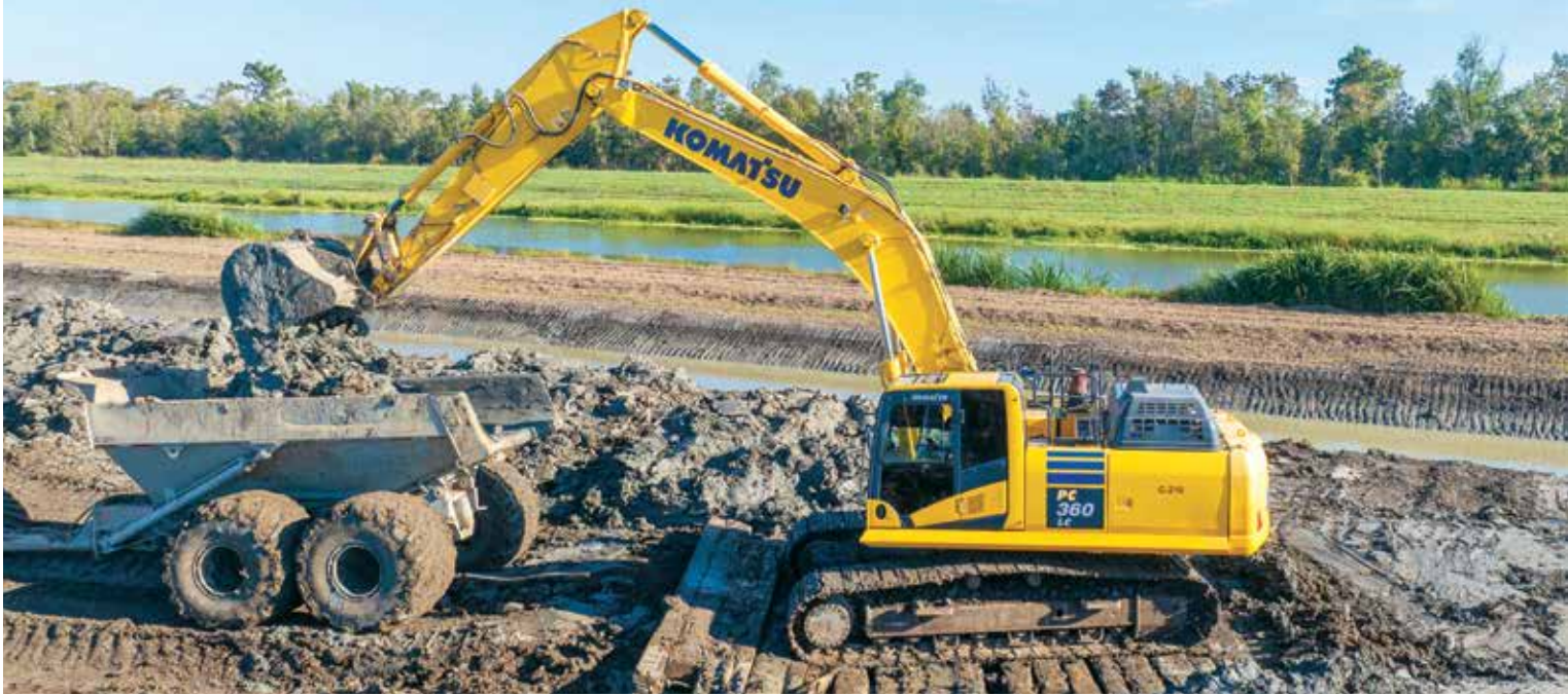
An Onshore Materials operator loads dirt on a levee project with a Komatsu PC360LC excavator.
